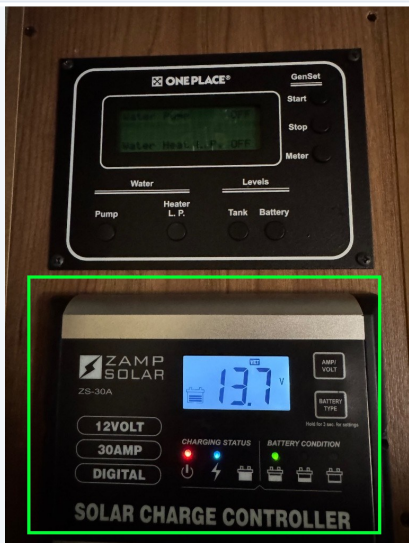
Solar Charge Controller
